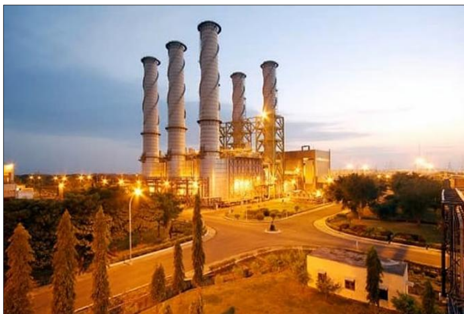
Image 1. File Photo of the Enron Power Project. Source: PSUWatch
